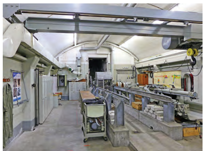
Fort Dailly: The workshop for the T1 15cm gun installation with the base station of the turret funicular
